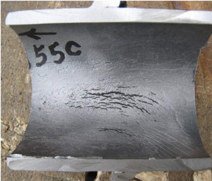
Figure 1. Stress-assisted corrosion cracking in the tube ID at the smelt box attachment.
