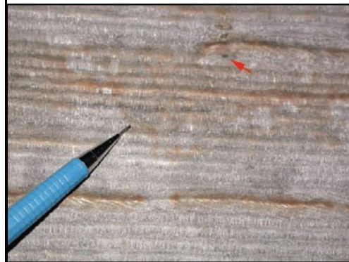
Type 309L Stainless Steel SAW Severe Corrosion Carbon Steel Exposure at Arrow
