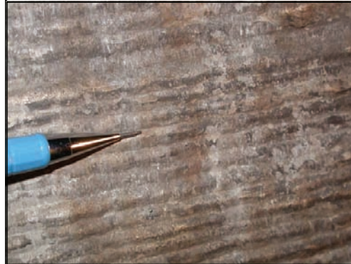
Type 309L Stainless Steel SAW Severe Deterioration (Replacement Needed)
