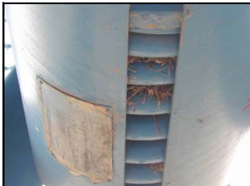
Figure 2. Closer View of Constant Support Hanger Fouled by Nesting Birds
