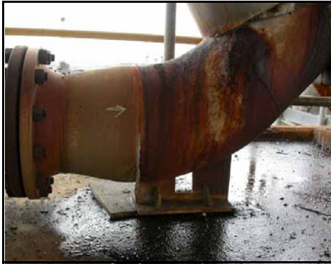
Figure 4. Slide Plate Displays a Dislodged HDPE Pad
