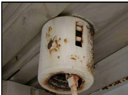
Figure 3. Variable Support Hanger Displaying Severe Corrosion
