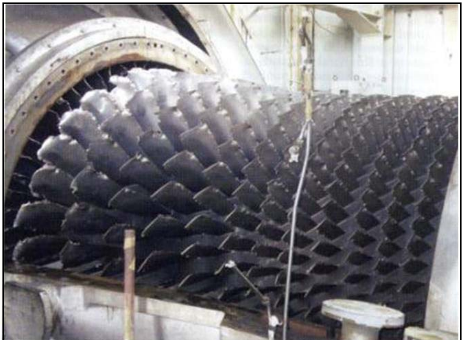
Figure 1. Failure of a first-row blade showing the damage to every stage of the compressor.
