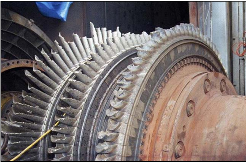
Figure 2. No bucket was left unscathed I this Frame 6 Turbine failure.
