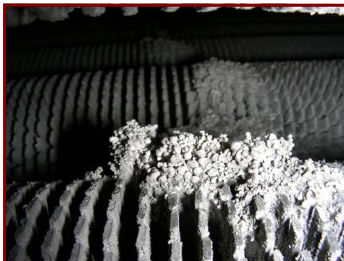
Figure 3. Deposits on the cook water tubes.
