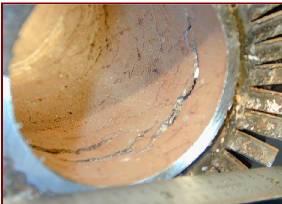
Figure 1. Multiple cracks on this stainless steel feedwater pre-heater tube actually started on the OD of the tube.
