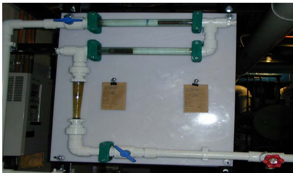
Figure 1. Corrosion Coupon Rack.
