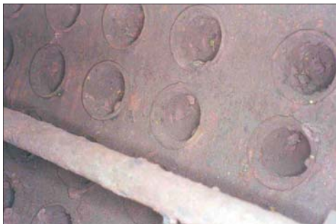
Figure No.1. Oxygen Pitting in Steam Drum.
