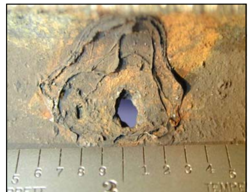
Figure 2. Typical Oxygen Pit.
